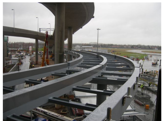
Photo of ATS ULTra PRT Track at Heathrow
